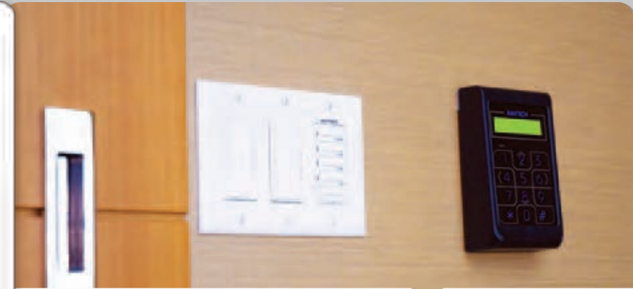
“Stand-alone proximity access control system”
