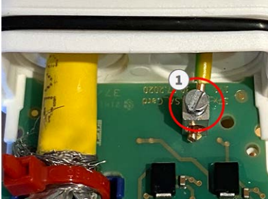
Fig. 28: Ground wire connected to terminal
