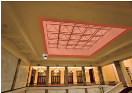
Skylight protection at Public facility / Warehouse
