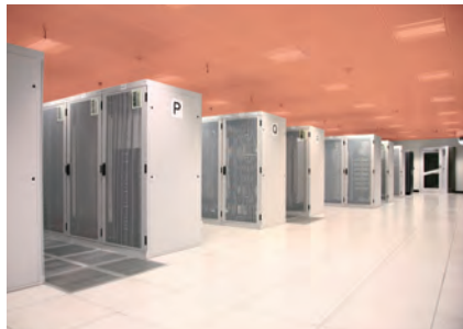
Ceiling protection at Data center
